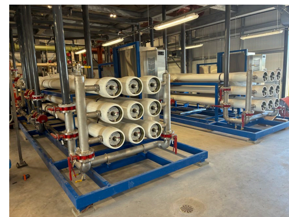
The two nanofiltration skids and associated piping had also been installed.
