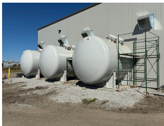
The three greensand filters had been installed.
